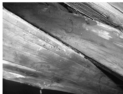
Figure 2.4.b. – House on Kogălniceanu street no. 6, Cluj-Napoca – position of rafter compared to the horizontal longitudinal element of the bracing system
