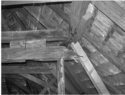
Figure 5.1. – Unprofessional interventions in the roof structure with baroque character of the Bădeni, Cluj county Unitarian church
