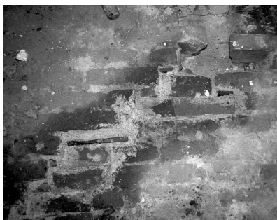
Figure 5.5.a. – Vault rebonding executed by specialised craftsmen employed by the general contractor – Tileagd, School with Classes I-VIII;
