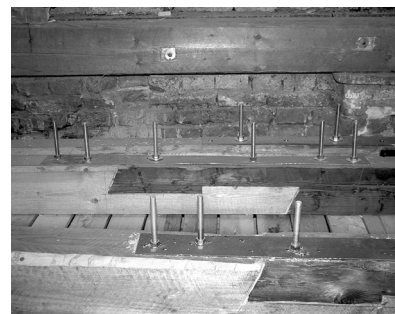
Figure 5.5.c. – The same continuation detail executed properly and in high quality, respecting the project.
