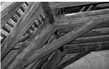
Figure 2.3.a. Compound rafter – counterbrace – straining beam joint, house on Kogălniceanu street no. 6, Cluj-N.
