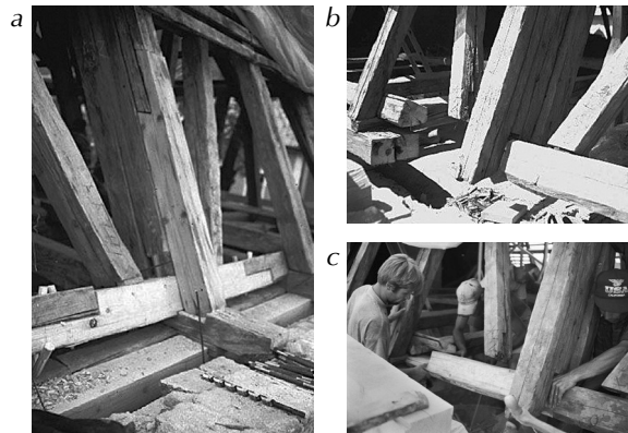
Figure 5.2. a-b-c – Minimal interventions, replacing portions of biologically degraded elements – Bethlen College, ACTT 2000; (TTF+IHBC).
